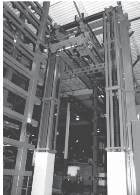
ASRS being set up in the plant. This handles sand cores for a buffer system for casting.
